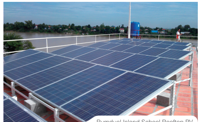
Rumdual Island School Rooftop PV (Source: Lawson Transworld)
