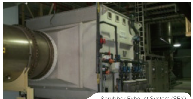
Scrubber Exhaust System (SEX)
