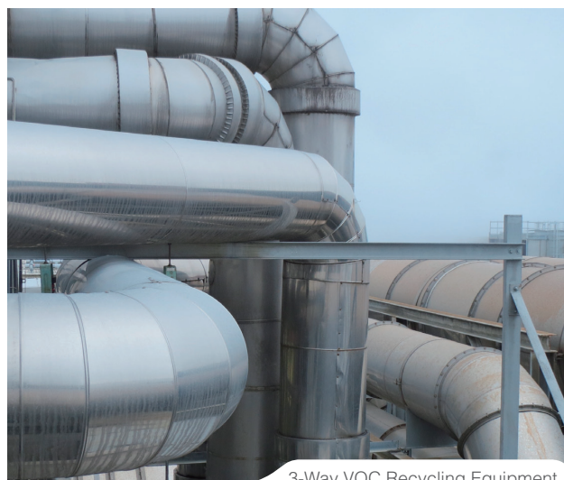
3-Way VOC Recycling Equipment (Source: Green Factory Label, 2013)
