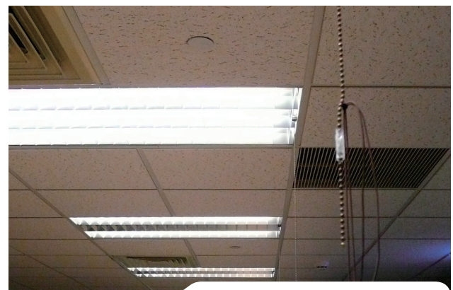
UMC String Switches for Office Lights
