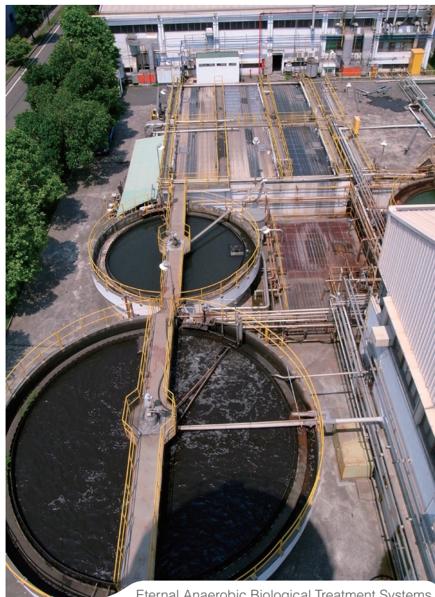
Eternal Anaerobic Biological Treatment Systems (Source: Green Factory Label, 2013)
